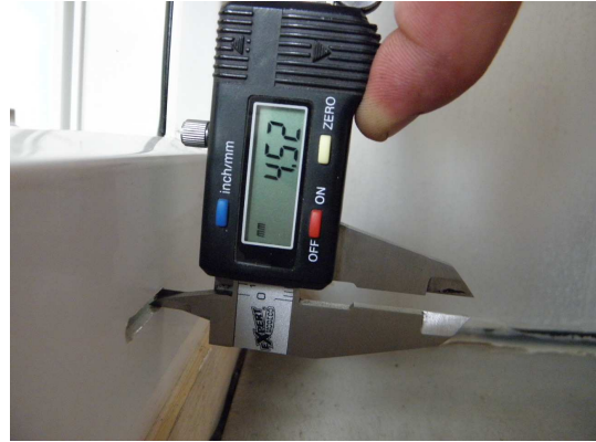
Picture 8 Rebate drainage
