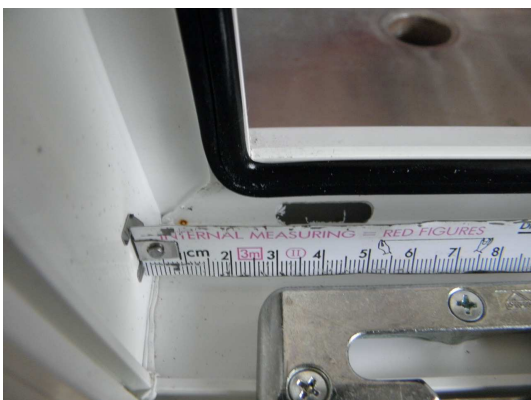
Picture 5 Rebate drainage
