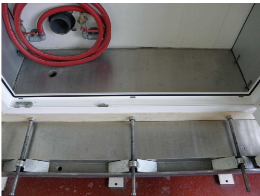
Picture 3 Rebate drainage
