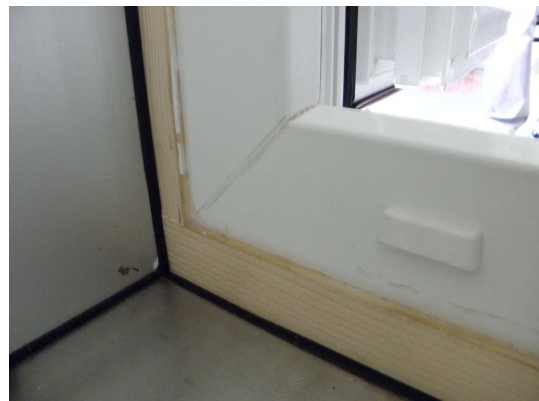
Picture 4 Rebate drainage
